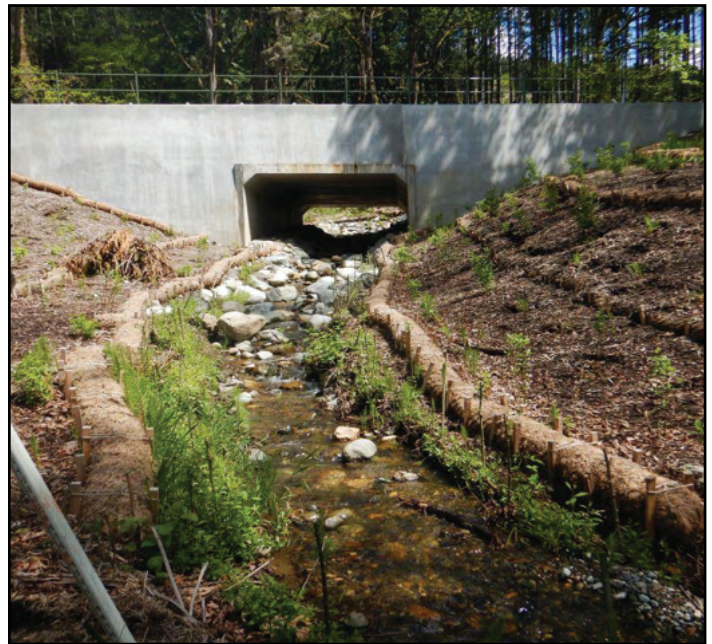
Figure 16. New 3-sided concrete water crossing structure is 80.5 ft in long and 16 ft wide.
