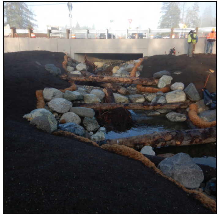
Figure 28. The new crossing is a 19 ft span by 5.6 ft rise concrete box culvert. The design reach immediately downstream of the new culvert is constructed of hardened step pools to connect the flat gradient of the headwater plateau where the project is located down a steep embankment to a wetland downstream. Juvenile salmonids were observed migrating through the step pools in May 2023.
