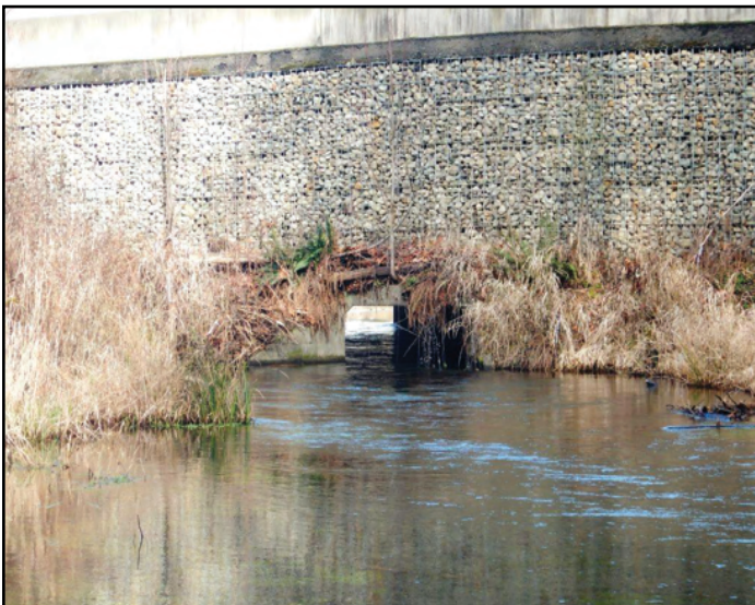
Figure 19. The structure removed was a 6 ft span by 5 ft rise concrete box culvert.
