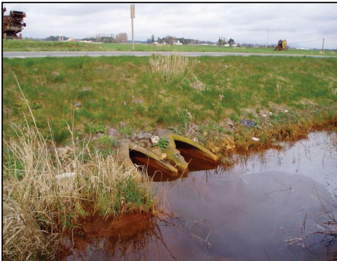
Figure 7. The old crossing under SR 546 consisted of two round 2 ft diameter concrete culverts.
