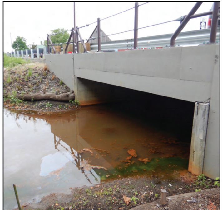
Figure 8. The new crossing is a 45 ft span by 7.5 ft rise concrete box culvert, providing fish passage to 0.64 miles of rearing habitat.
