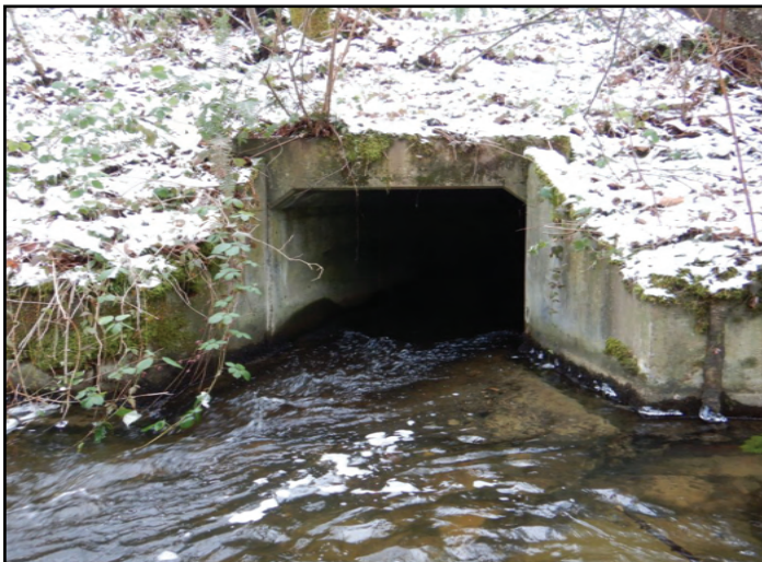
Figure 5. The previous structure was a 5 ft square concrete box culvert by 425 ft long. It was a total barrier due to slope and low flow depth.
