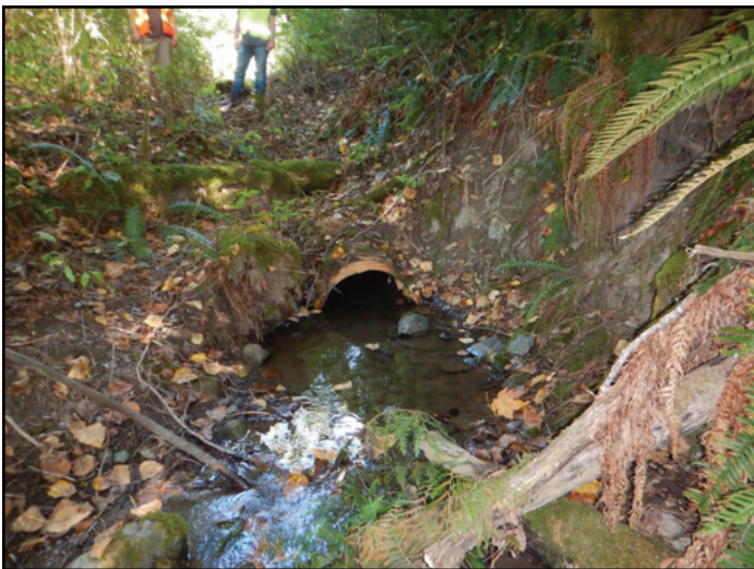
Figure 17. The old crossing was a 2 ft diameter and 300 ft long mixed material pipe with a slope of 3.05%. This crossing was considered a total barrier due to slope. Before construction, the upstream channel flowed along SR 20 in a ditch and under 3 driveways that were each fish passage barriers.
