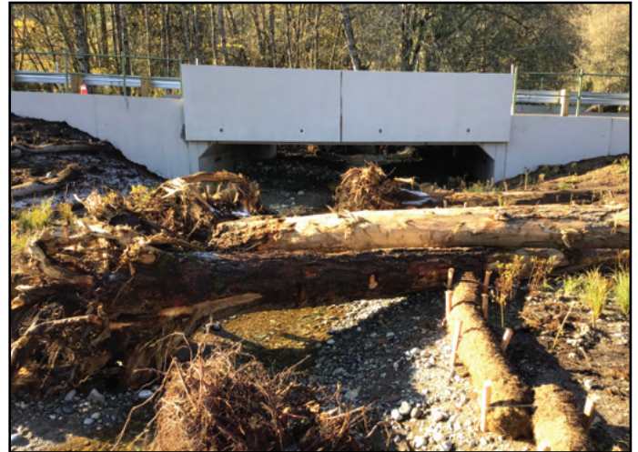
Figure 14. The new crossing is a 26 ft span by 10.6 ft rise concrete culvert and is 35 ft long.
