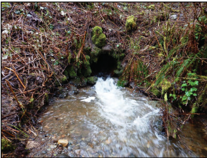
Figure 15. The previous crossing was a 2.5 ft diameter by 145 ft long corrugated metal pipe culvert which was a barrier to salmonid passage due to both inadequate water depths and unacceptably high water velocities. Before this barrier removal project, this site was also frequently obstructed with debris and posed a maintenance problem.
