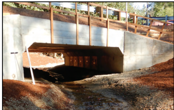
Figure 24. The new lower crossing is a 18.9 ft span by 14 ft rise concrete box culvert. The new upper crossing is also a concrete box culvert, 18.3 ft span by 14 ft rise.
