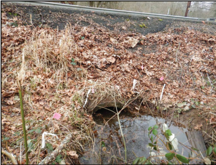
Figure 13. The undersized crossing consisted of a round 3 ft diameter 41 ft long concrete pipe. This structure was a partial barrier due to the slope of the pipe exceeding fish passable standards.
