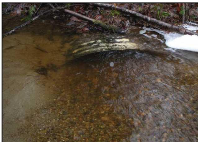
Figure 21. The old crossing for 996794 was a 2 ft diameter culvert and the old crossing for 996795 was a 3 ft diameter corrugated aluminum culvert.
