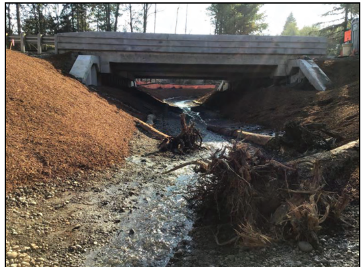
Figure 22. The new crossing under Chico Way NW is a 41.8 ft bridge, restoring access to 0.8 miles of habitat for chum, coho, steelhead, coastal and resident cutthroat trout.
