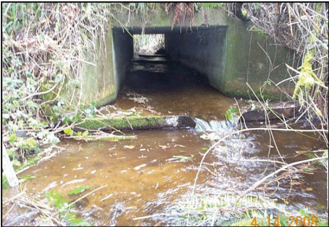
Figure 23. Both old crossings were 6 ft span by 4 ft rise concrete box culverts with an attached fishway consisting of 4 steel baffles inside the culvert and bed controls downstream of each structure. The lower culvert was a barrier due to an excessive water surface drop. The upper was a barrier due to insufficient water depth after the bed controls failed.
