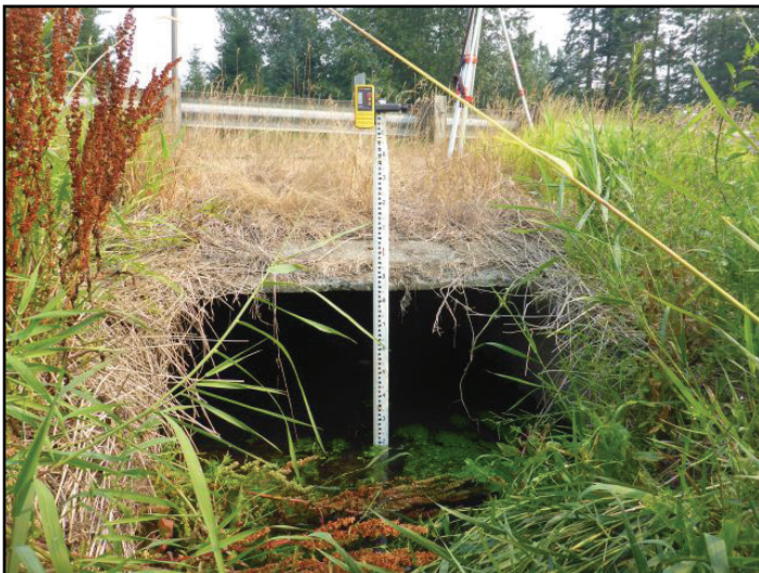
Figure 11. The old crossing was a 6 ft span by 4 ft rise concrete culvert.
