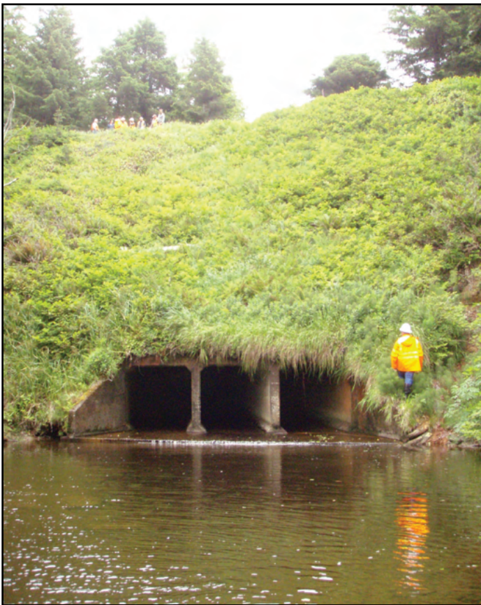
Figure 25. The old crossing was a triple cell concrete box culvert with each cell measuring 6 ft span by 6 ft rise that was retrofitted in 1998 with a baffled fishway in each cell to facilitate fish passage. The fishway was assessed as a barrier due to excessive water surface drop at the outlet.
