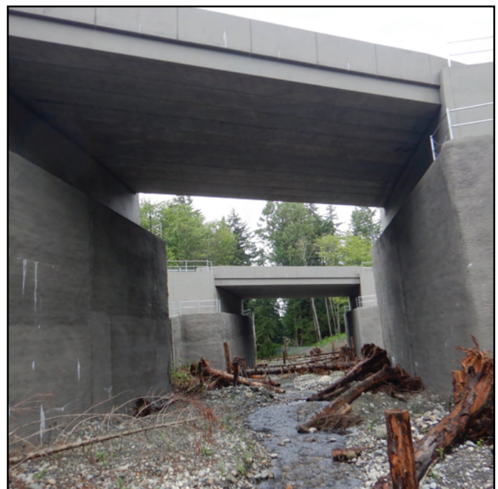
Figure 6. The barrier was replaced with two 44 ft span bridges with a 64 ft setback wall in the median, restoring access to 2 miles of upstream habitat for chum, coho, steelhead, kokanee from Lake Padden, and coastal and resident trout.
