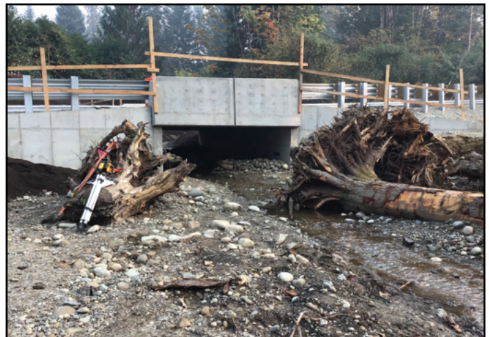
Figure 18. The new crossing is a 13 ft wide by 9.6 ft rise by 40 ft long concrete box culvert. The project design realigned the stream to avoid passing through the 3 barrier driveway culverts.
