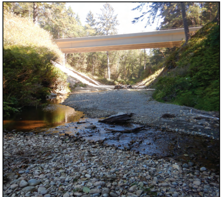
Figure 26. The new crossing is a 208 ft bridge. Adult coho salmon were observed spawning upstream of the new bridge in November 2022.
