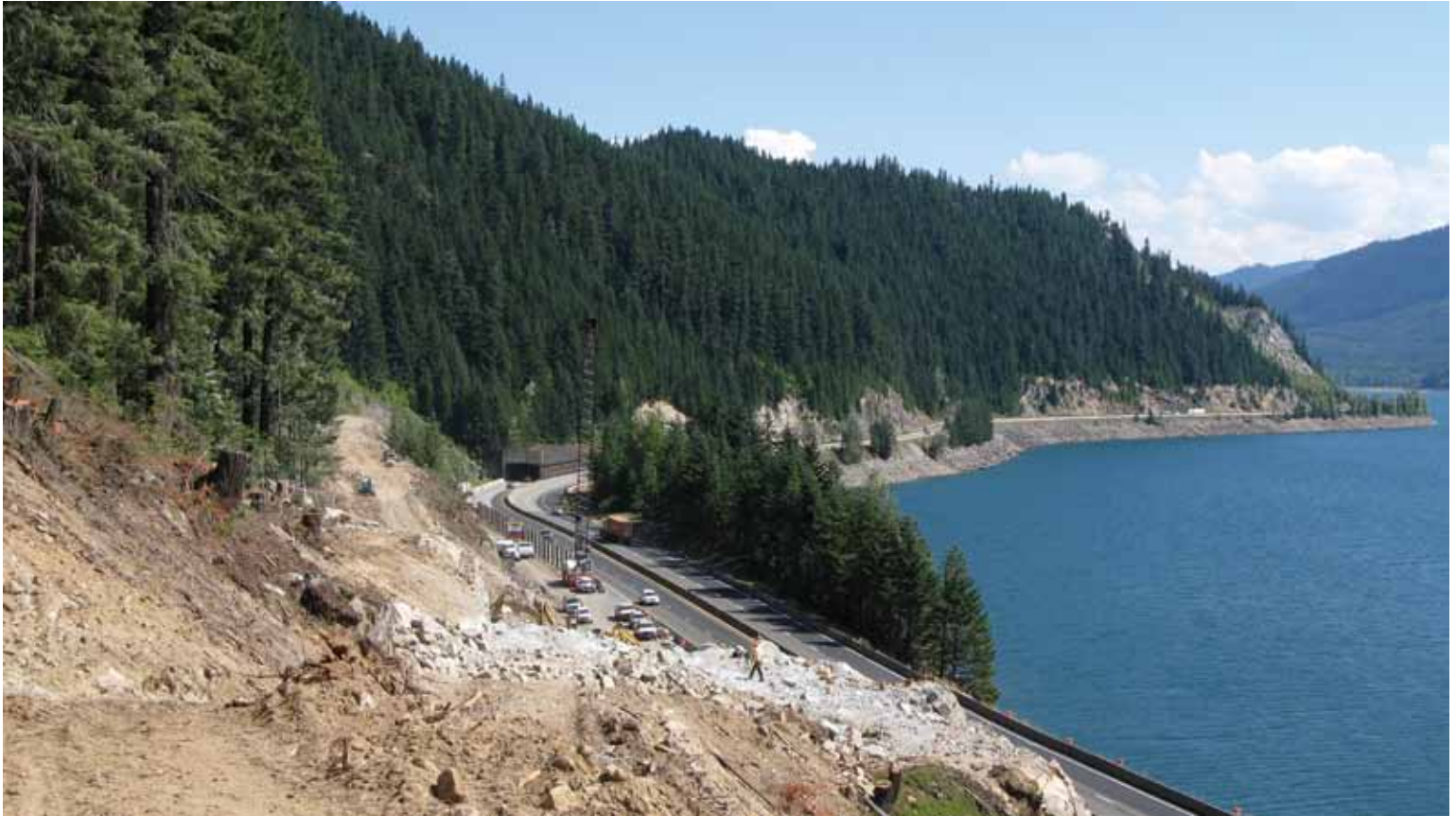
WSDOT will temporarily close I-90 at sunset for up to one hour for rock blasting work, Monday through Thursday
