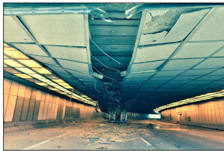
Damage to tunnel ceiling.
