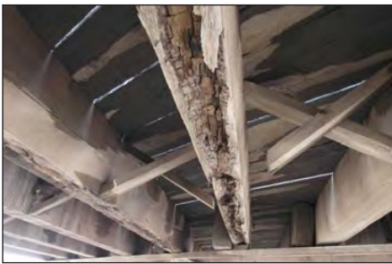
Rotted timbers of the support structure.
