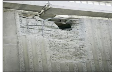
Concrete is chipping and flaking off girders and piers.
