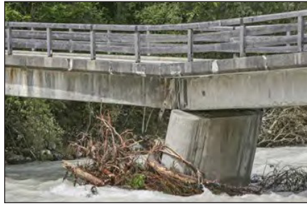
Drift debris build-up at bridge pier. This can cause undermining of footings.
