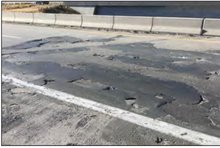
Concrete is chipping off the deck and portions of the expansion joint are missing.
