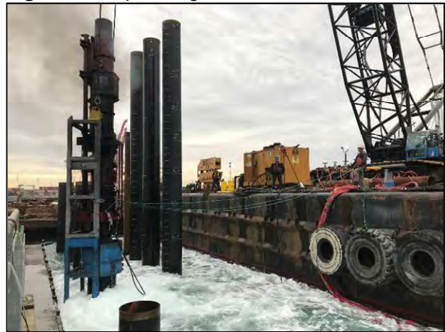
Figure 5.2 Operating Bubble Curtain
